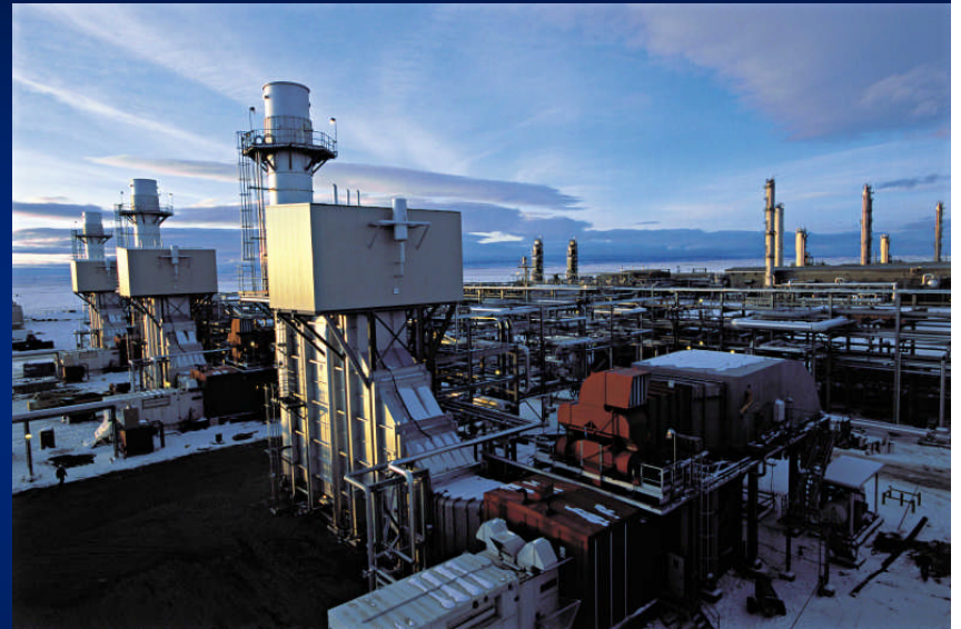
LaBarge AGI Cogen Wyoming, USA
