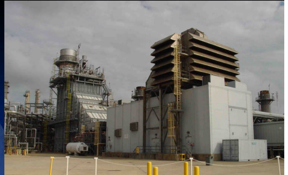
Baytown Train 4 100-MW Siemens v84.2 Baytown, TX USA
