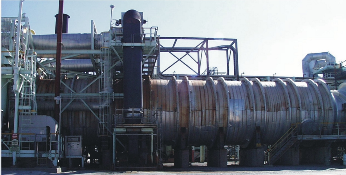
Sulfuric Acid Recovery Furnace
