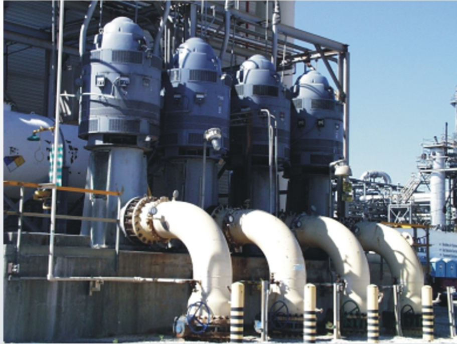
Cooling Tower Pumps for the Acrylates Area
